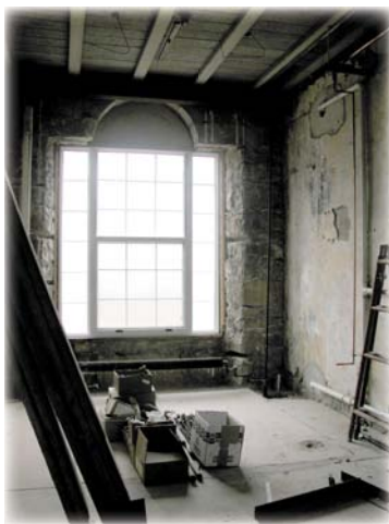
Part of the renovation of A-D involved installing energy-efficient windows throughout the building. The arches at the top of windows like this one will also be replaced, UIU Director of Operations Ron Crooker said. The arches were covered during the last renovation.
