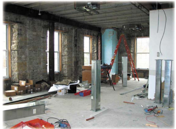
The second floor of A-D is in the midst of the renovation process. Seen here in early February, the floor had been gutted in preparation of new interior walls being erected.
